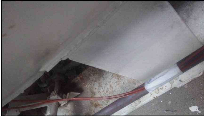
RTD sensor installed on LN2 fill line
